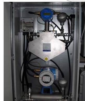
Picture shows the flow meter panel with ATEX rated Coriolis flow meters
