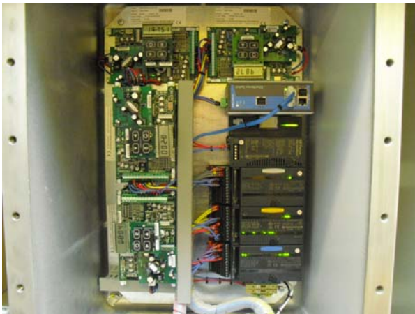
Picture shows the PLC Control installation within an ATEX Enclosure
